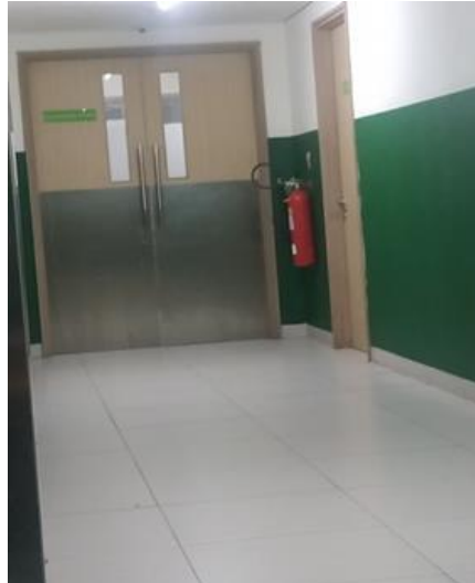
Figure 2. Fire Extinguisher at Employee Corridor in Harris Vertu Hotel [Source: Author, 2023]
